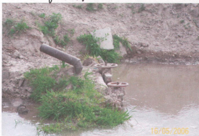
Riverside Canal Canal - supplemental water intake 5/16/2006 SH
