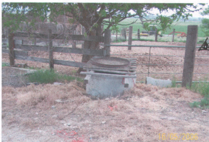
collection/control valves box for 63-21520 + 63-21521 5/16/06 SH
