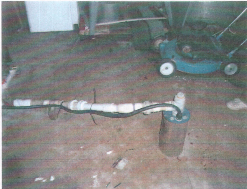
This photo shows the West well.
