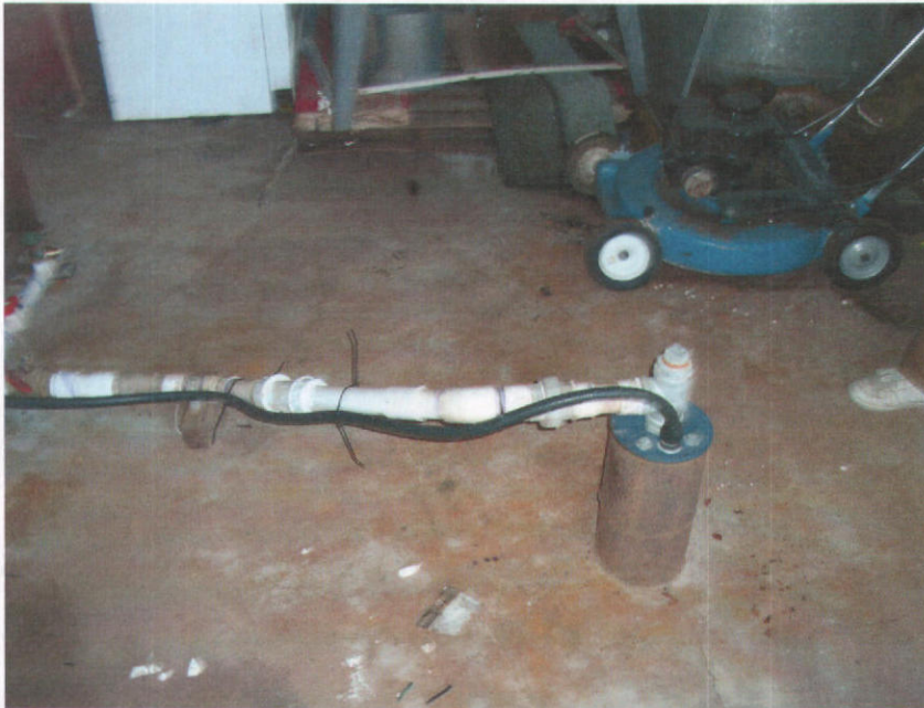
This photo shows the West well.
