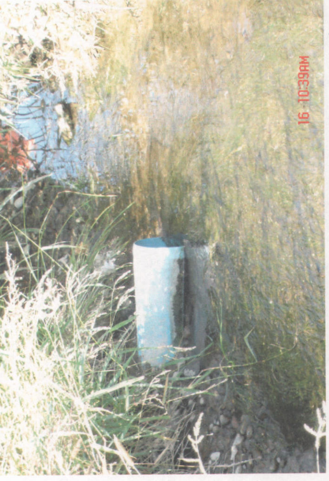
15in Pipe from head gate Across road.
