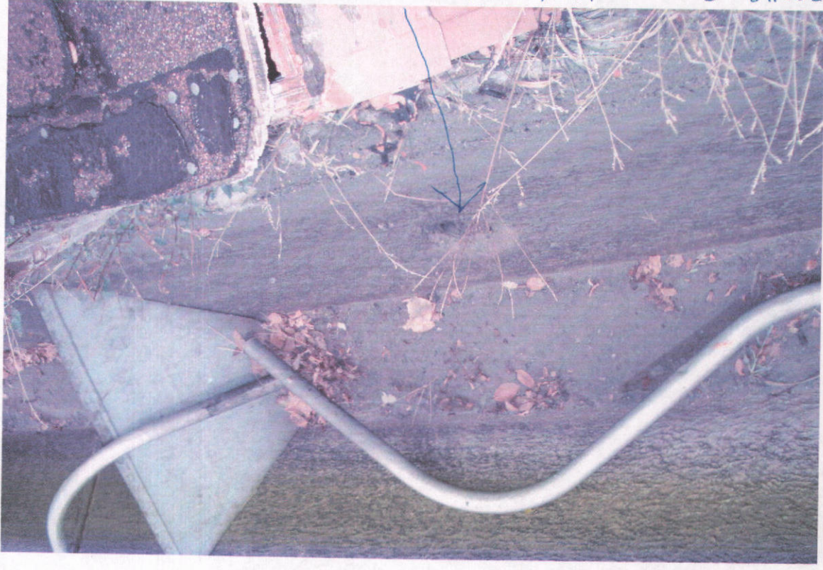
pic#3 Cement ditch with INlet From Pump
