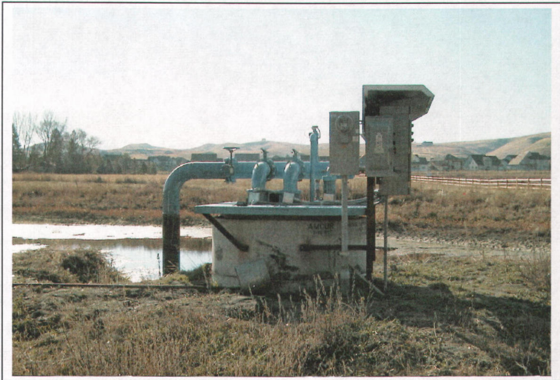
Photo 3: Distribution pond with re-lift water pumps. Piped into pressurized sprinkler irrigation system. View is to south in the SWNE, S31, T05N, R02E.
