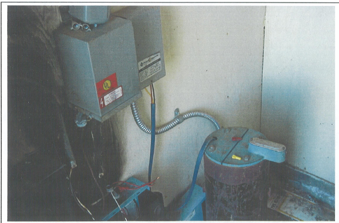
Photo 2. Inside of well house. Submersible pump is 1 HP, 8 inch casing.
