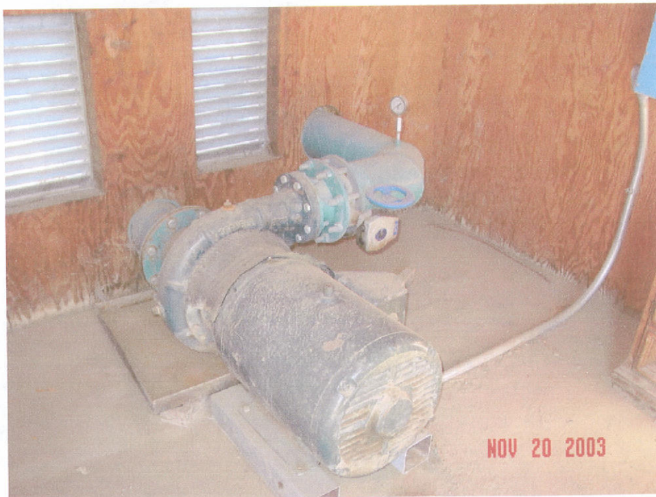
Second pump system inside pump house 63-26699
