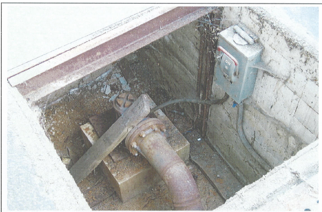
Photo 2. Well under grate. Casing cannot be seen however data from Mayne Pump Company shows a 14-inch casing with 5-inch out flow pipe. Located in the SWSENE, T03N, R02E, S10.
