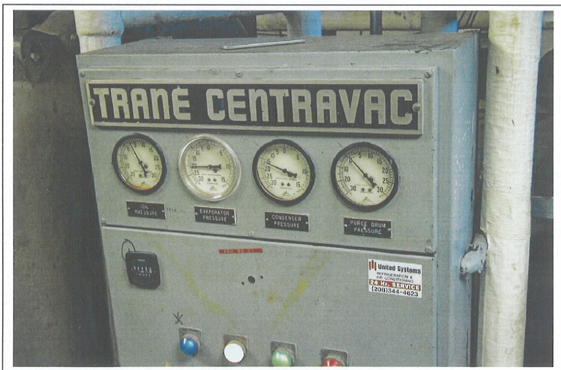
Photo 6. Type of system control, Trane Centravac.
