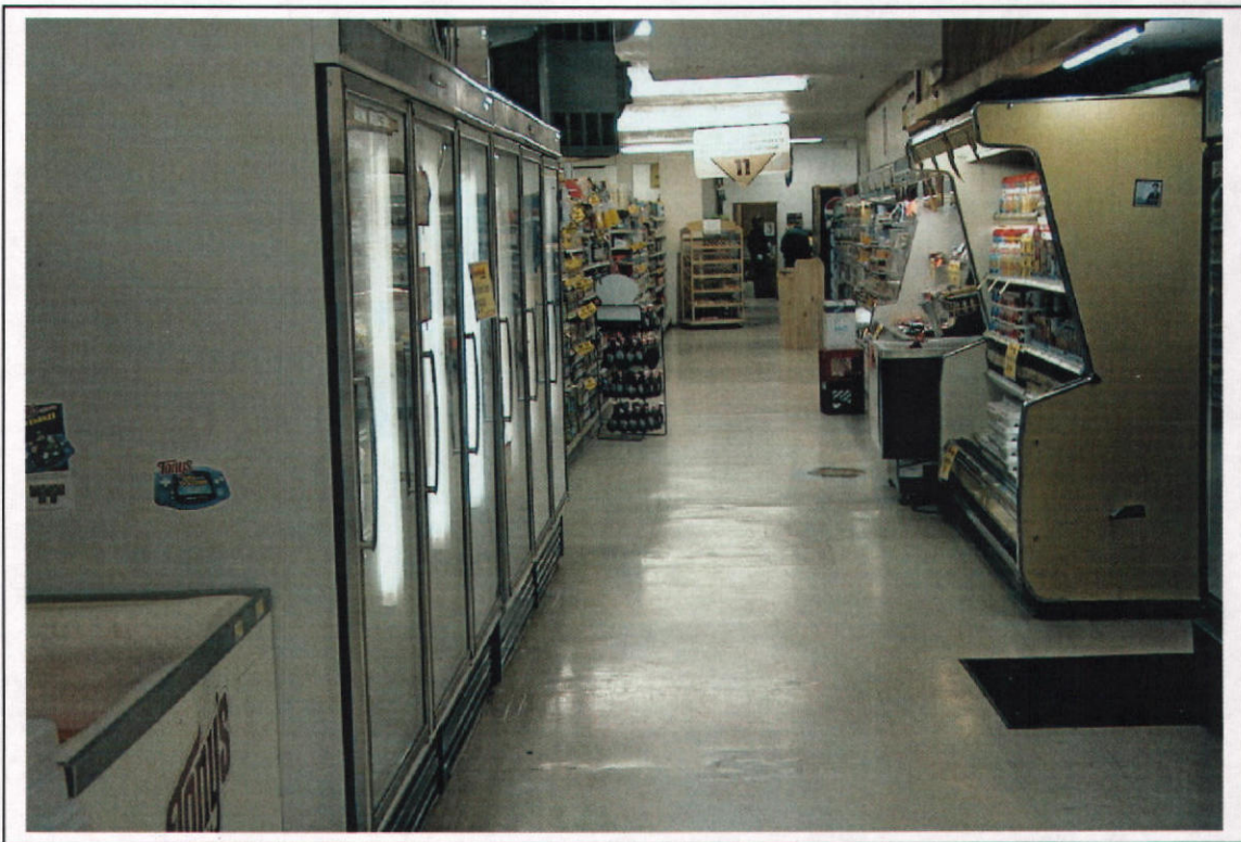
Photo 4: Store cooling units.
