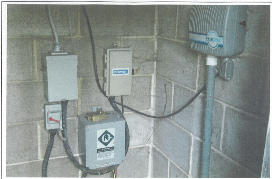
Photo 1. 63-19651 Field Exam 7/24/02. Photo's by RDH. Controls inside well house. Unknown HP of pump or size of casing. Casing is not visible, no HP information. No well log found.
