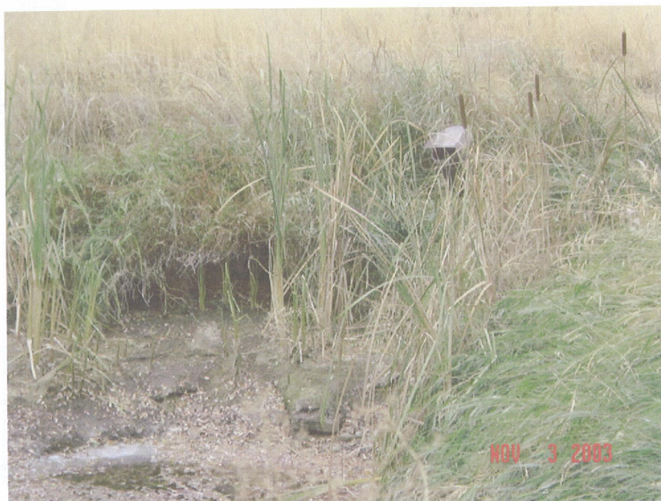
Pipe for delivery from well to pond
