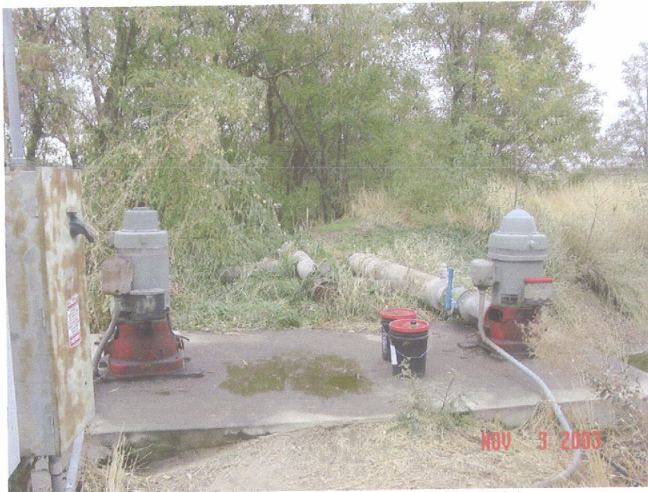
Pumps to send water from pond to fields
