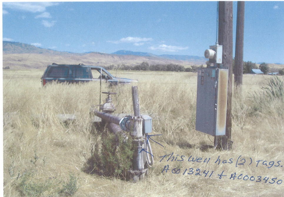
Picture # 21 8" Well with submergible pump
