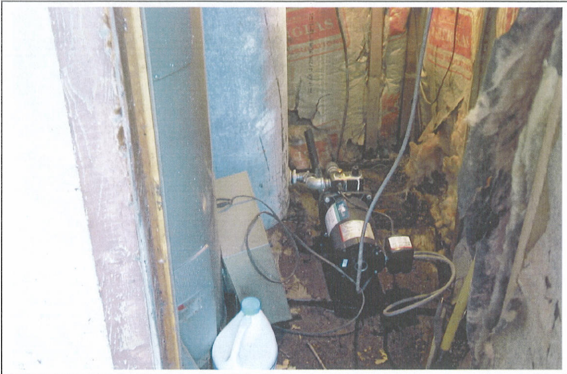
Photo 1. 63-17333 Field Exam 11/01/02. Photo's by RDH. View of well in well house, located on North side of Crawford's building as shown on photo 2. Property address is 2720 Fargo.
