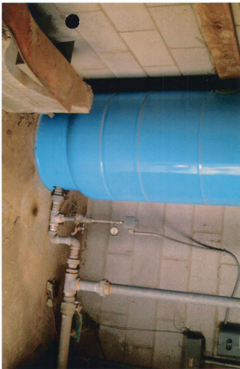
Inside well House
