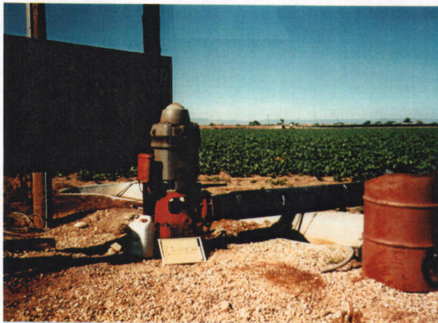
#1 Point of diversion and discharge pipe. Field in background is part of P/U.
