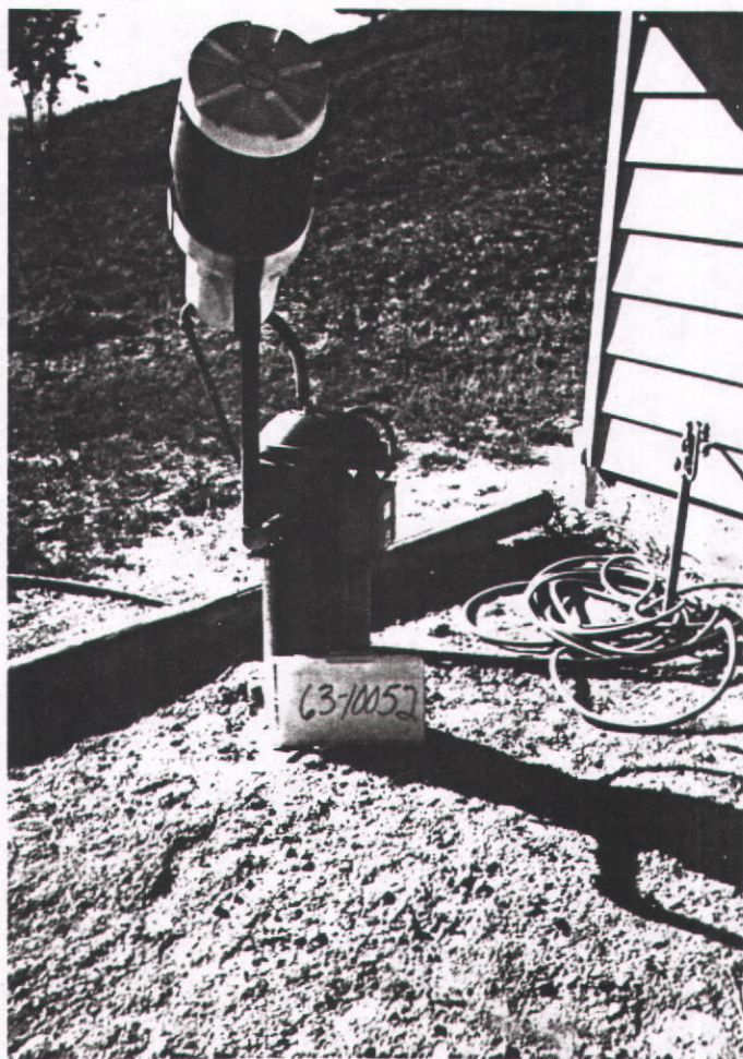
#2 P/D - Irrigation well.
