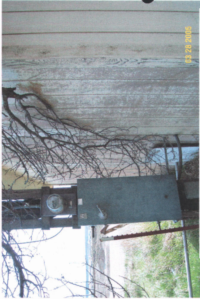
Pump power meter and panel—East side of pump house
