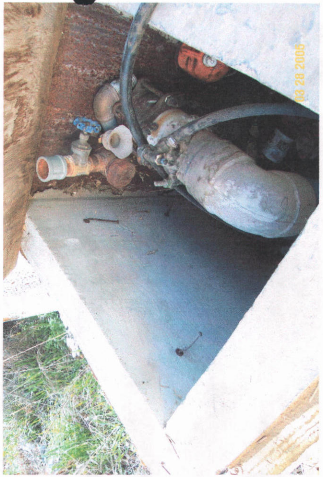
6" Outlet Pipe from Tank
