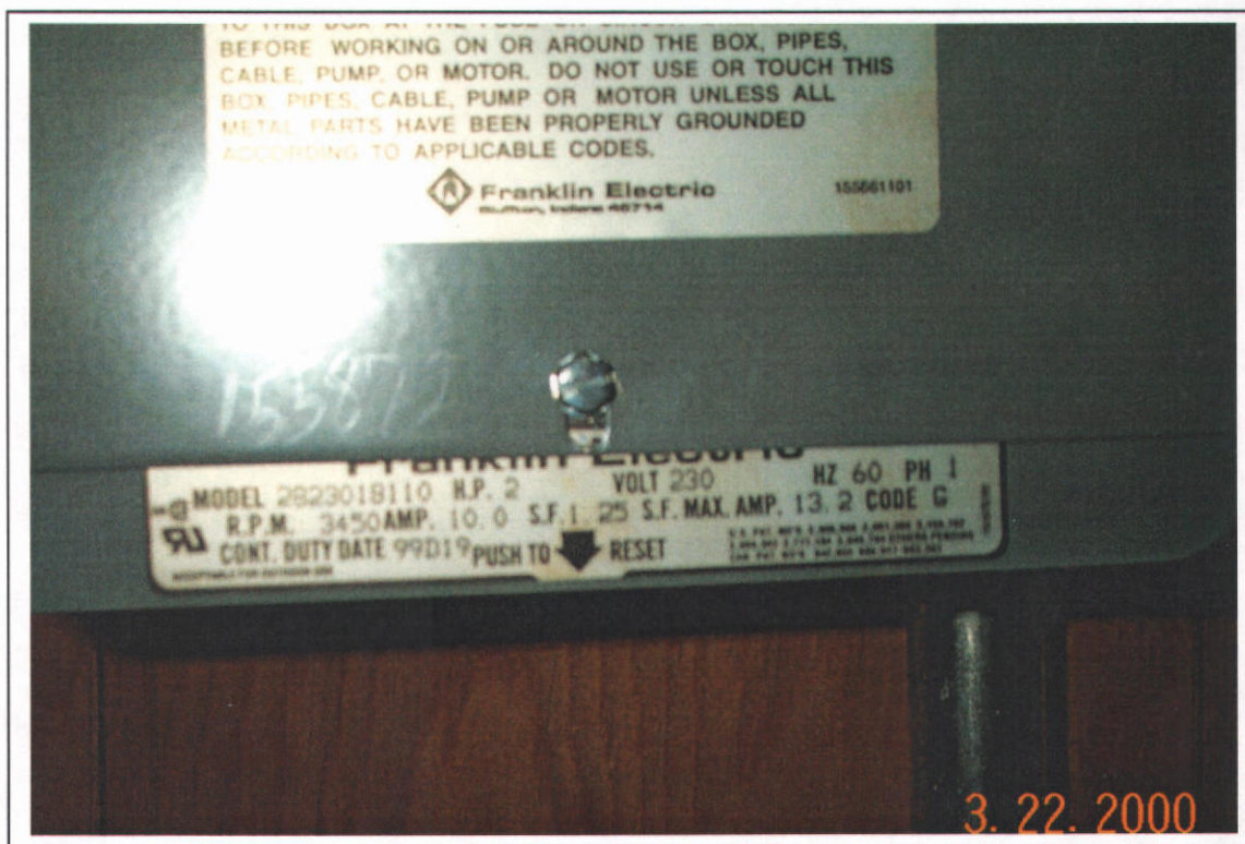
Photo 4: Photo by Intrepid Engineering Services showing pump data.
