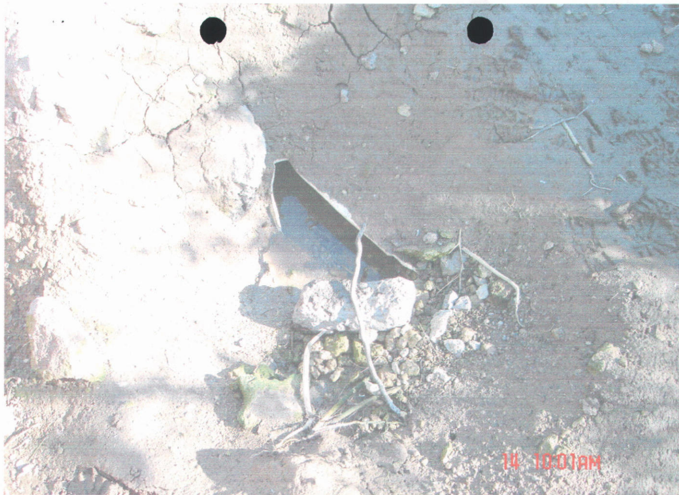
6 inch PVC Pipe from 3rd Pod
