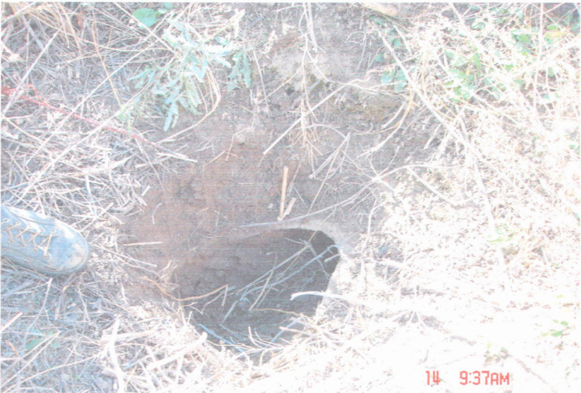
12 inch Culvert Seawing 1 Pod Pond
