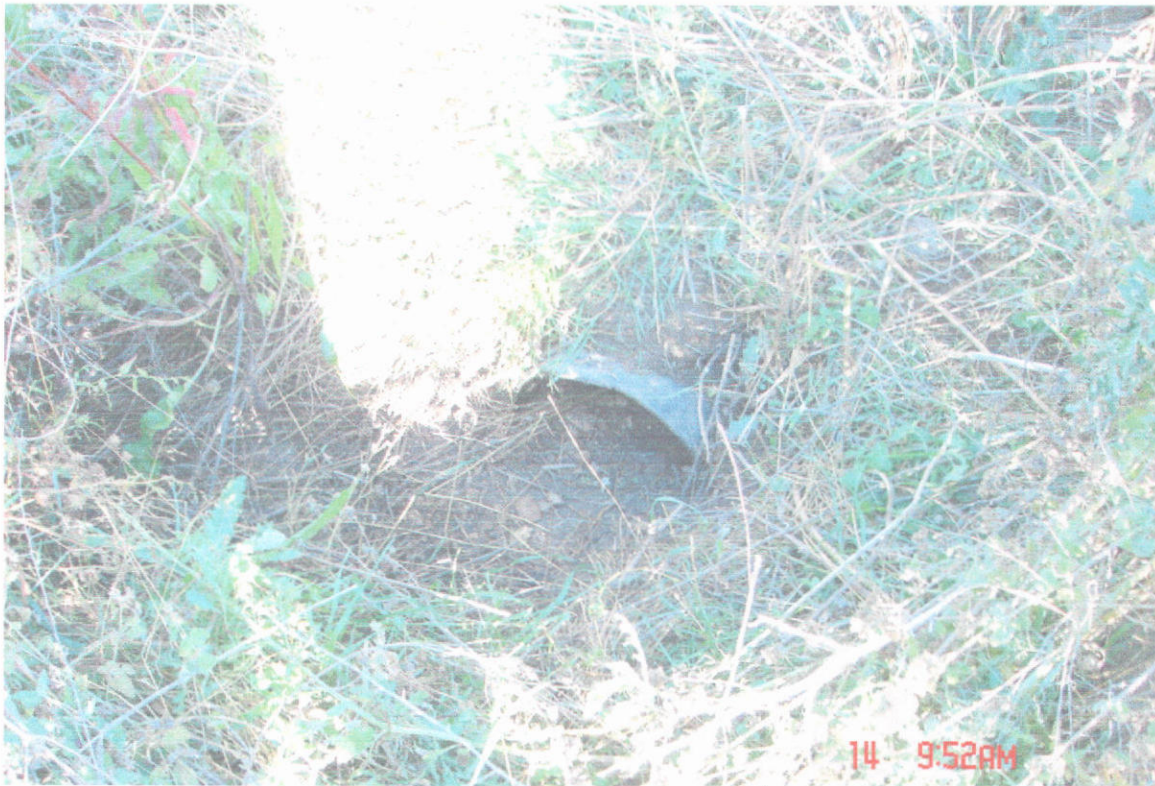
2nd Pod 12 inch culvert runs into Pond.
