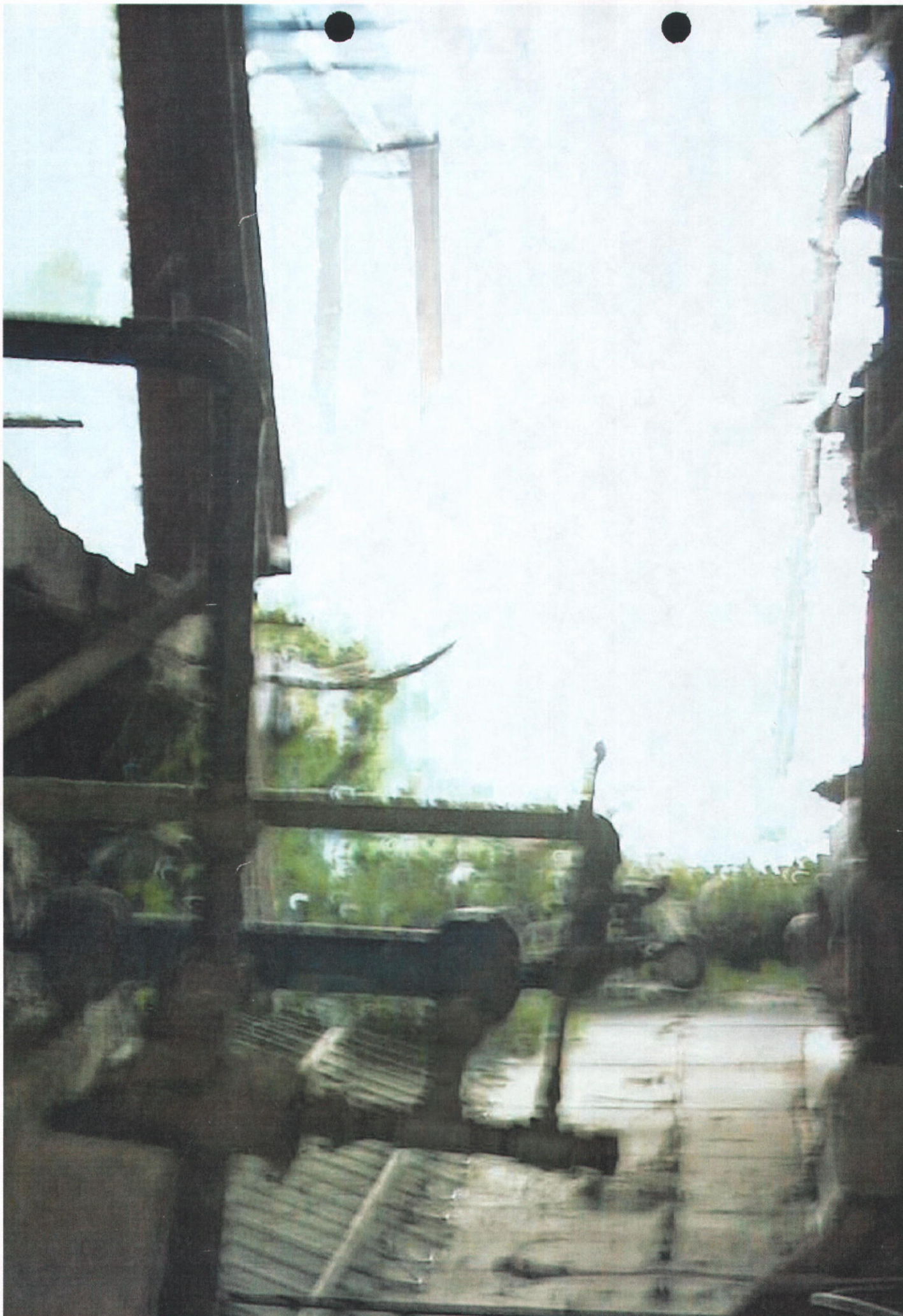
A63-5296 Waste Water 2HP 2" pump and lines
