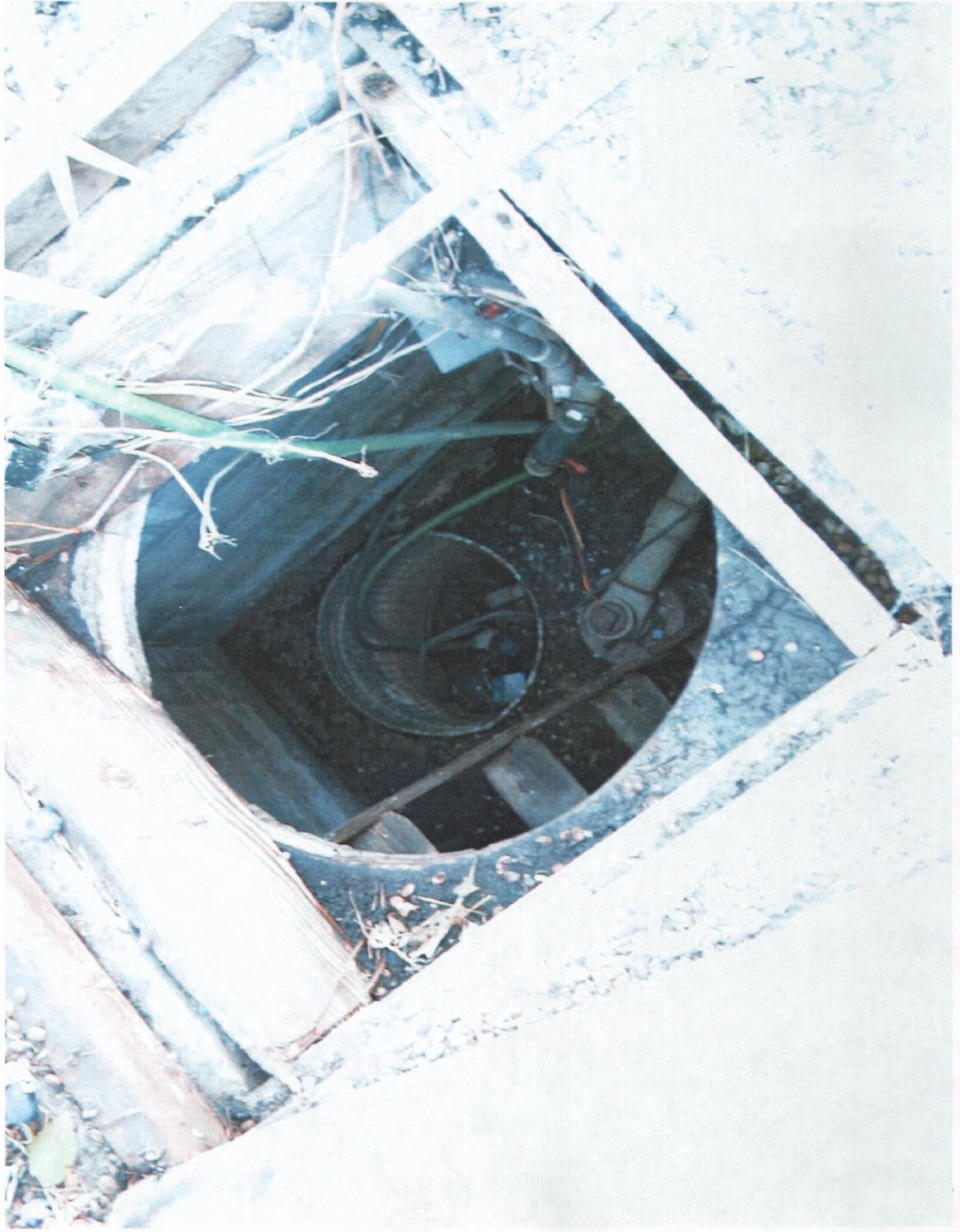
A63-5292 GW Well 2HP 2" pump and lines
