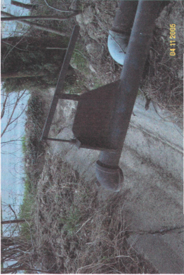
Outlet from pump into West Ditch looking East
