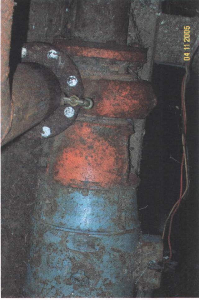
Centrifugal Pump 7.5 HP
