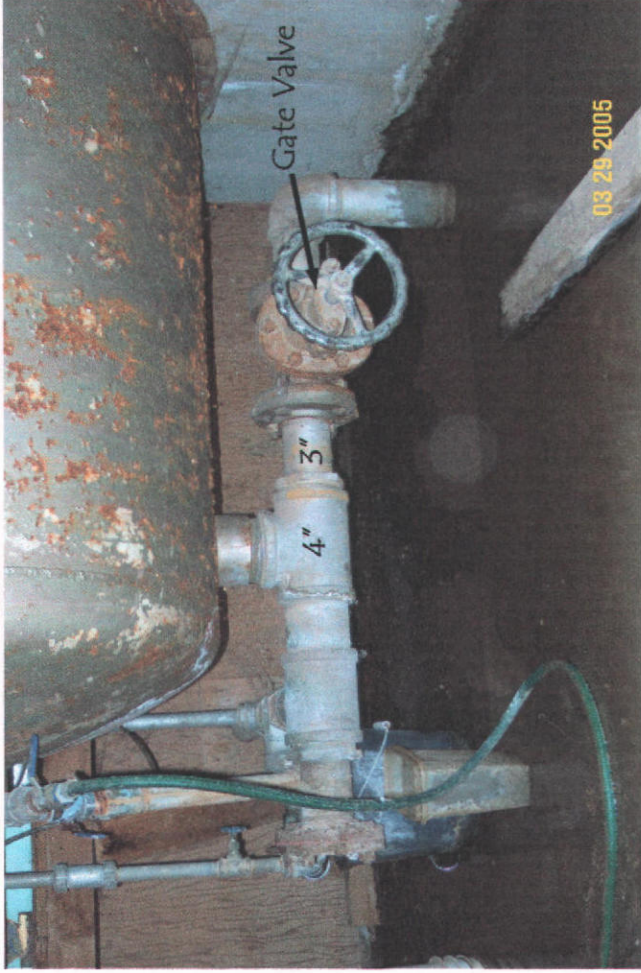
Outlet Plumbing from Pressure Tank
