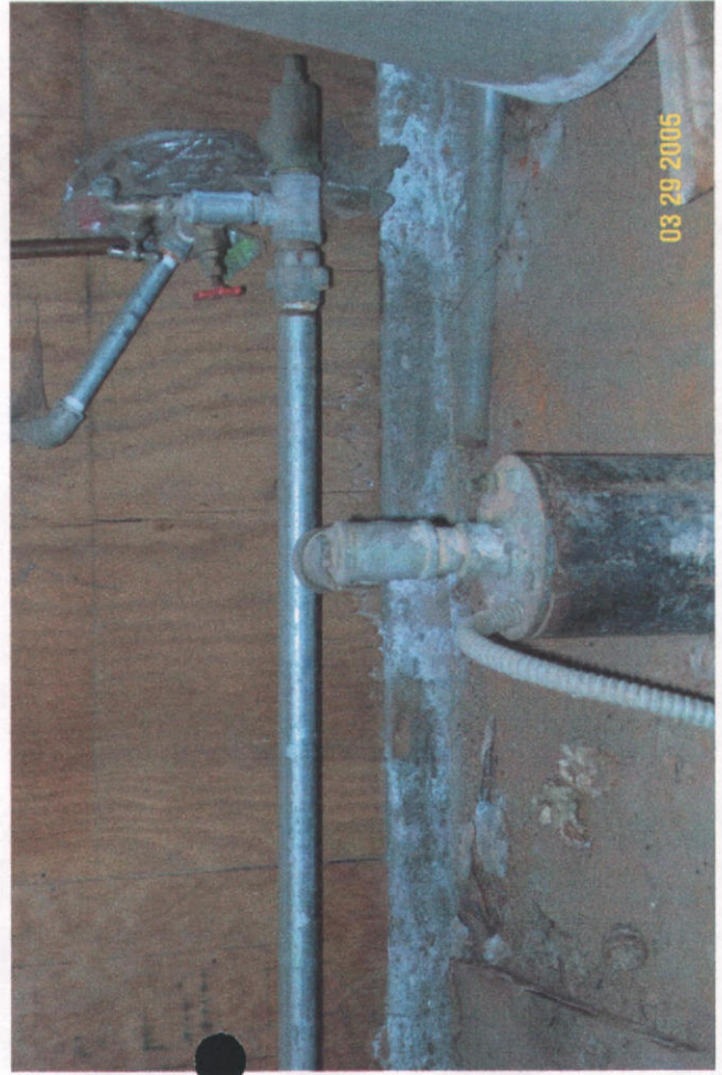
Pump disconnected from system—currently not in use
