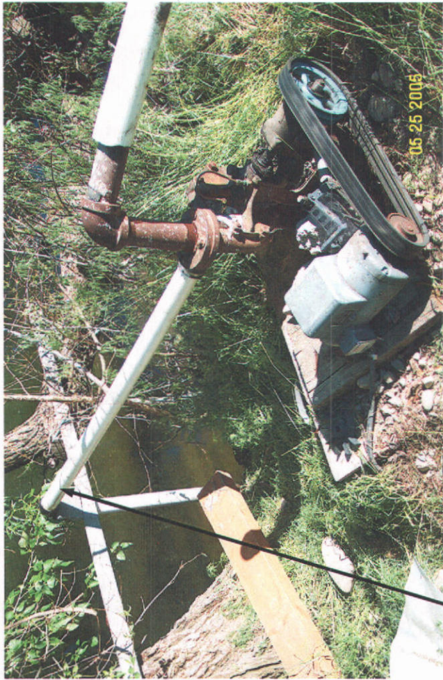
Pump Suction in South Fork of Boise River
