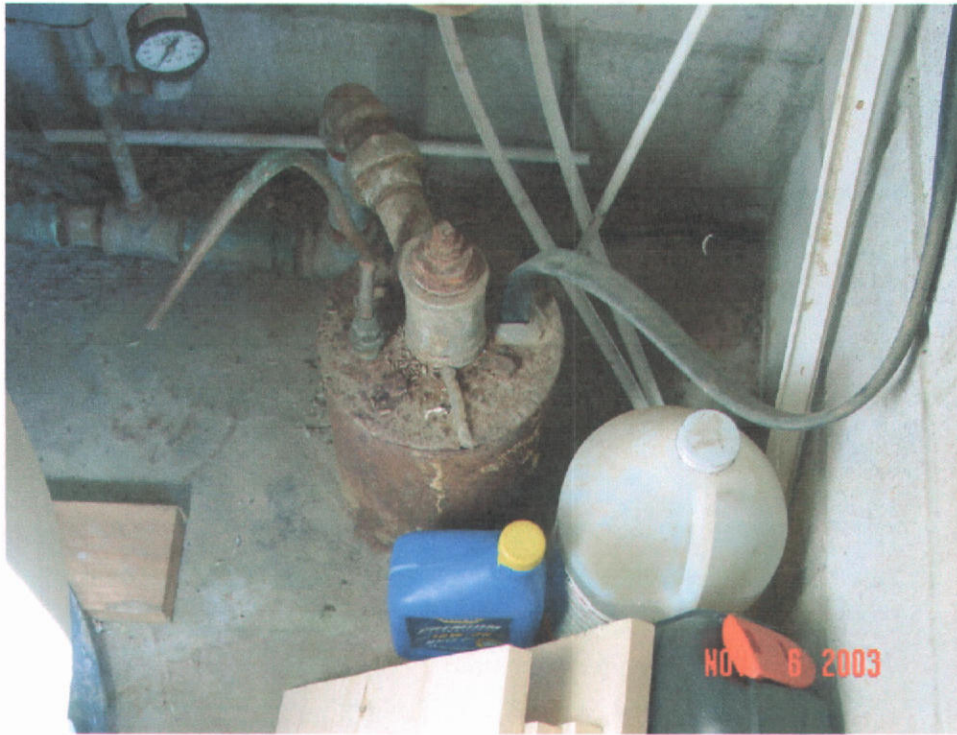
Well inside pump house.
