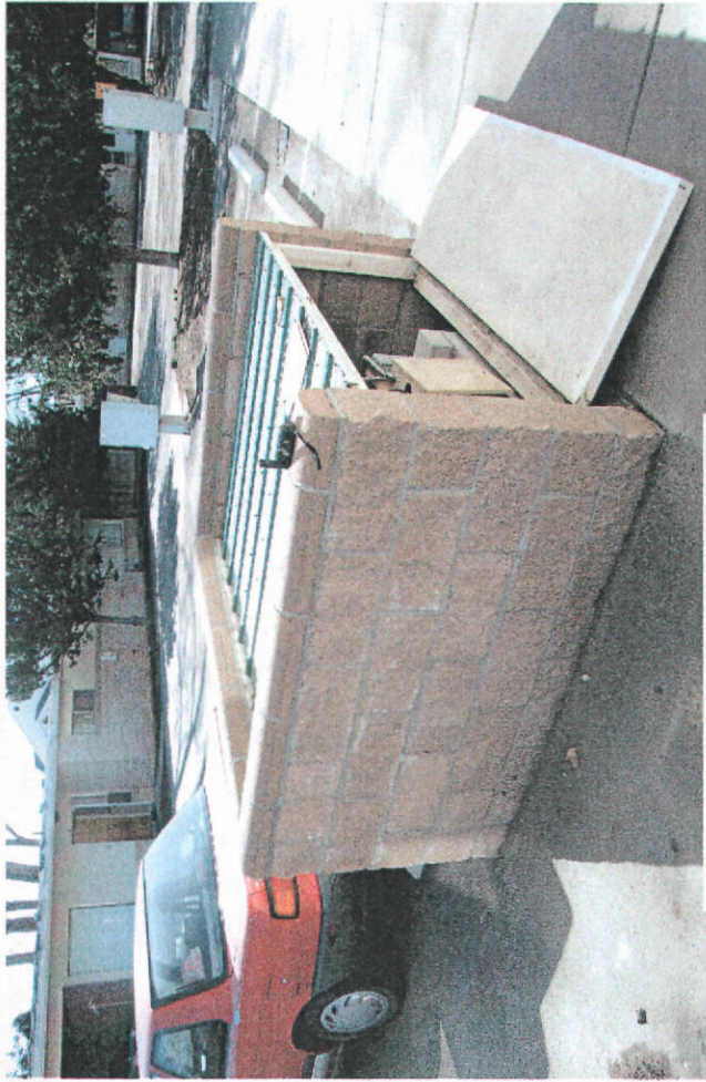
Pump #1, Looking Southwest
