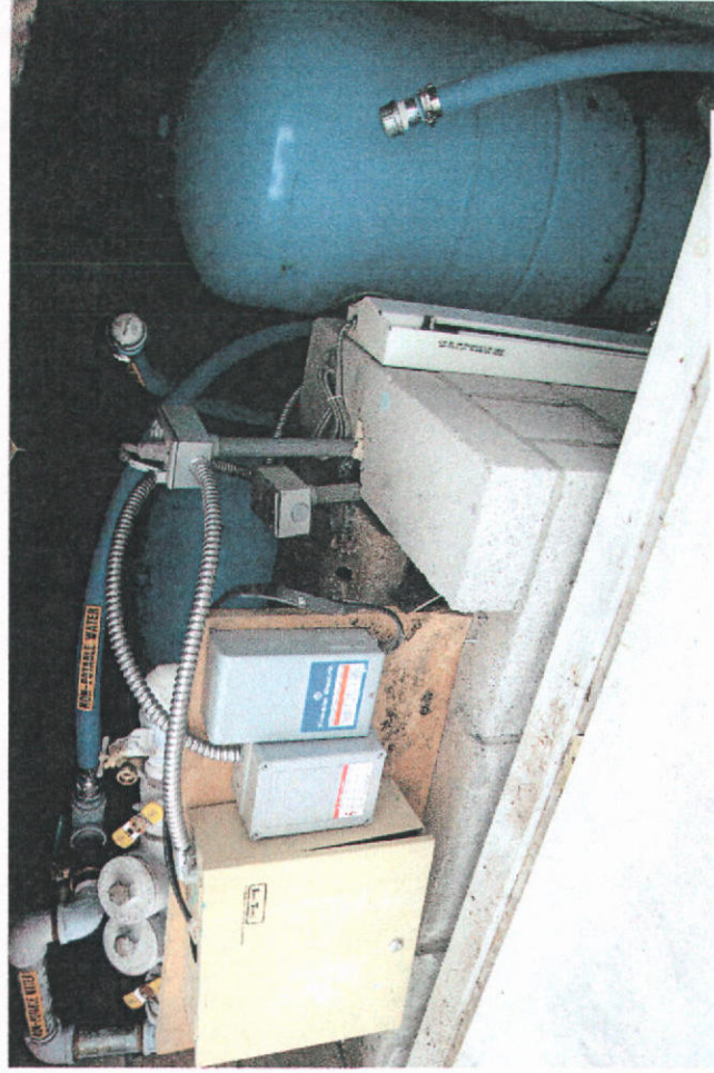
Pump #1, Pump and Sprinkler Controls
