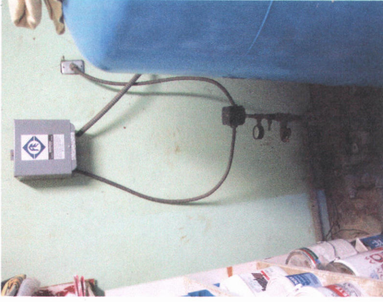
Pump #2, Pressure tanks & controls
