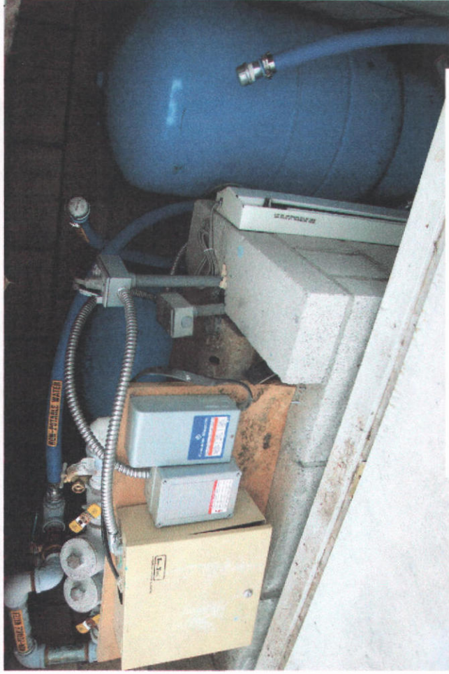
Pump #1, Pump and Sprinkler Controls
