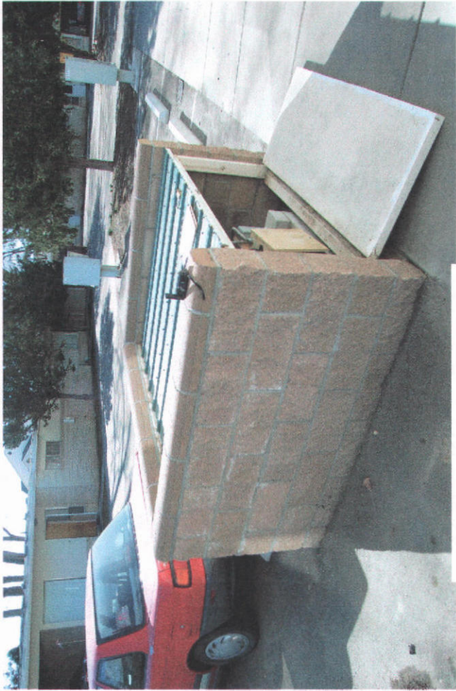
Pump #1, Looking Southwest
