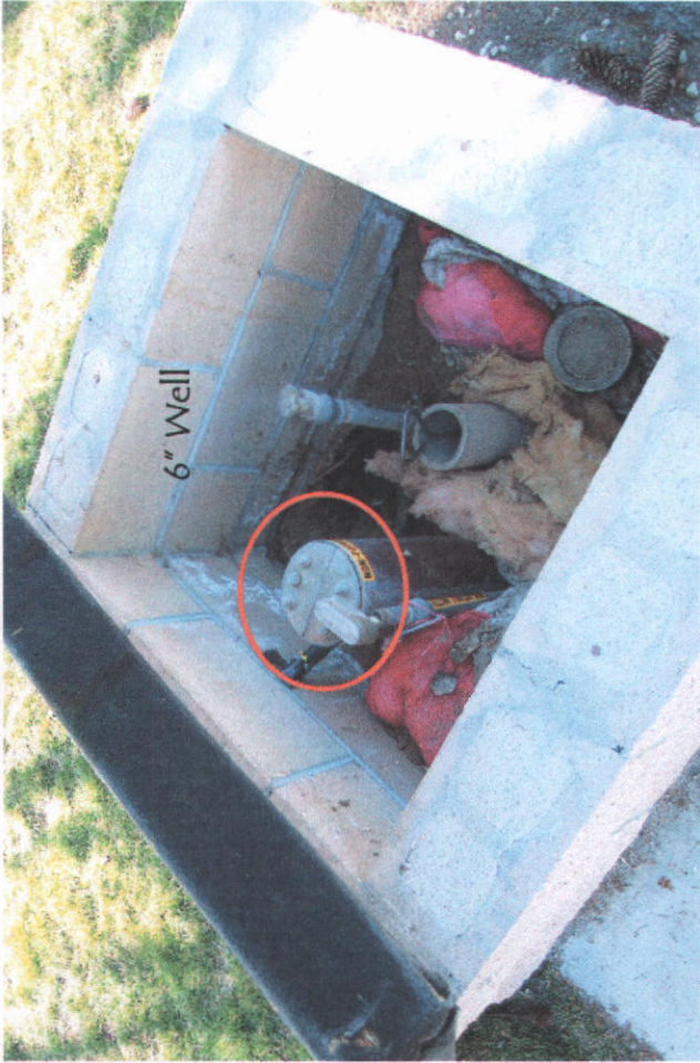
Well / Pump #2, looking West
