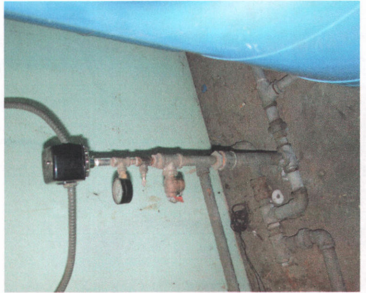
Pump #2 Plumbing, etc.
