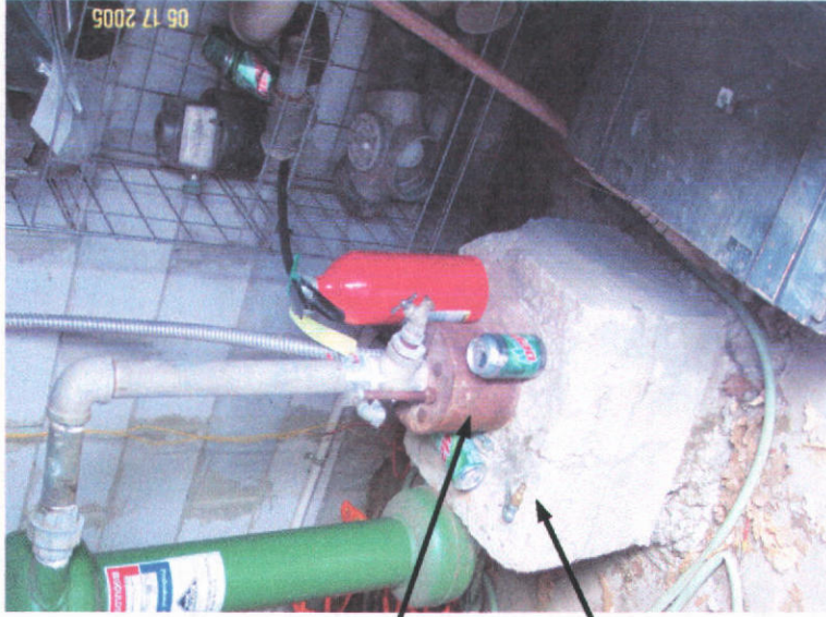
South Well Head 6" inside diameter
