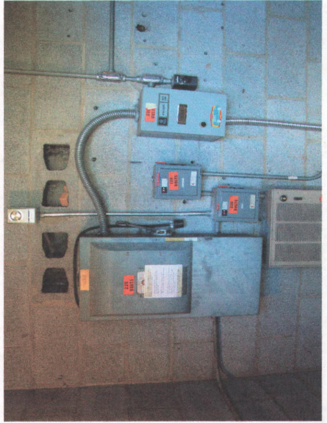
Electrical Control Panels for pump and controls
