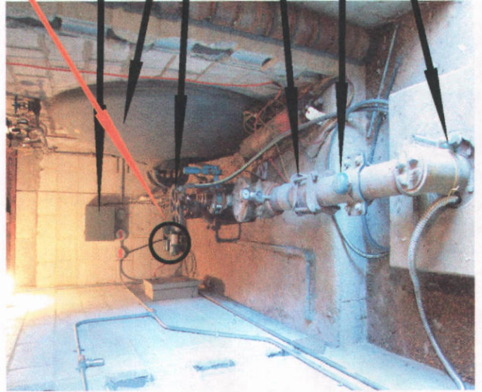
Air Compressor for pumping air into pressure tank
