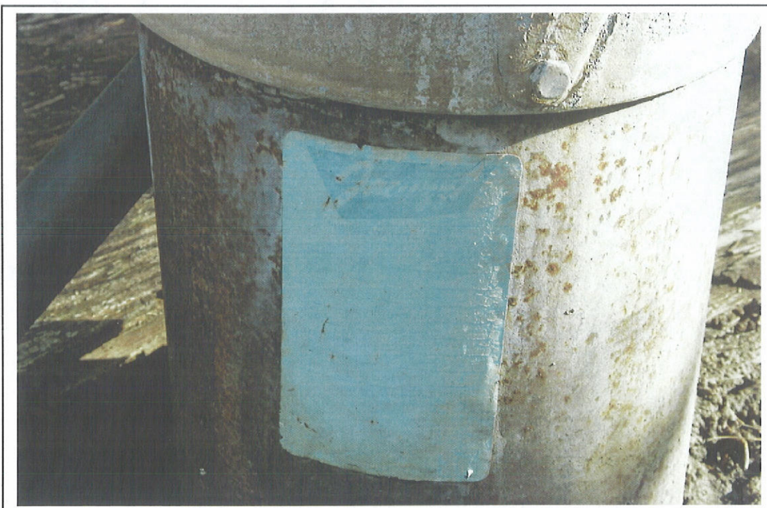
Photo 2. Close up view of tag on 8 " well with Jacuzzi pump. Could not read data.
