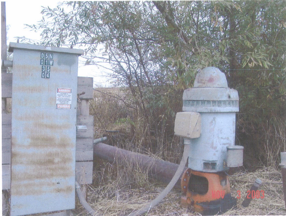
Pumping system facing NW.
