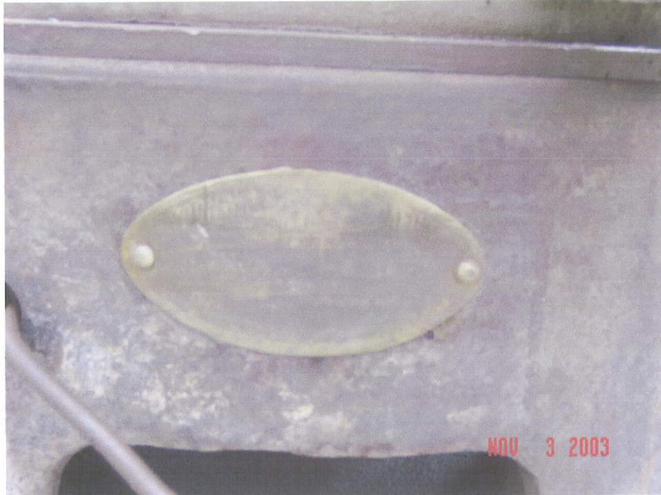
New well pump nameplate
