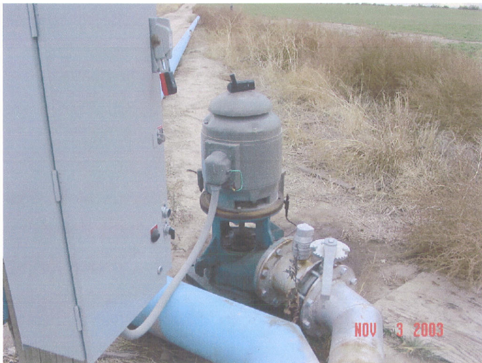
Original pumping system facing SW.
