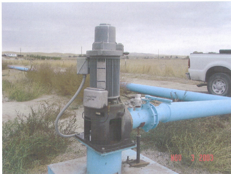
New pumping system facing S.
