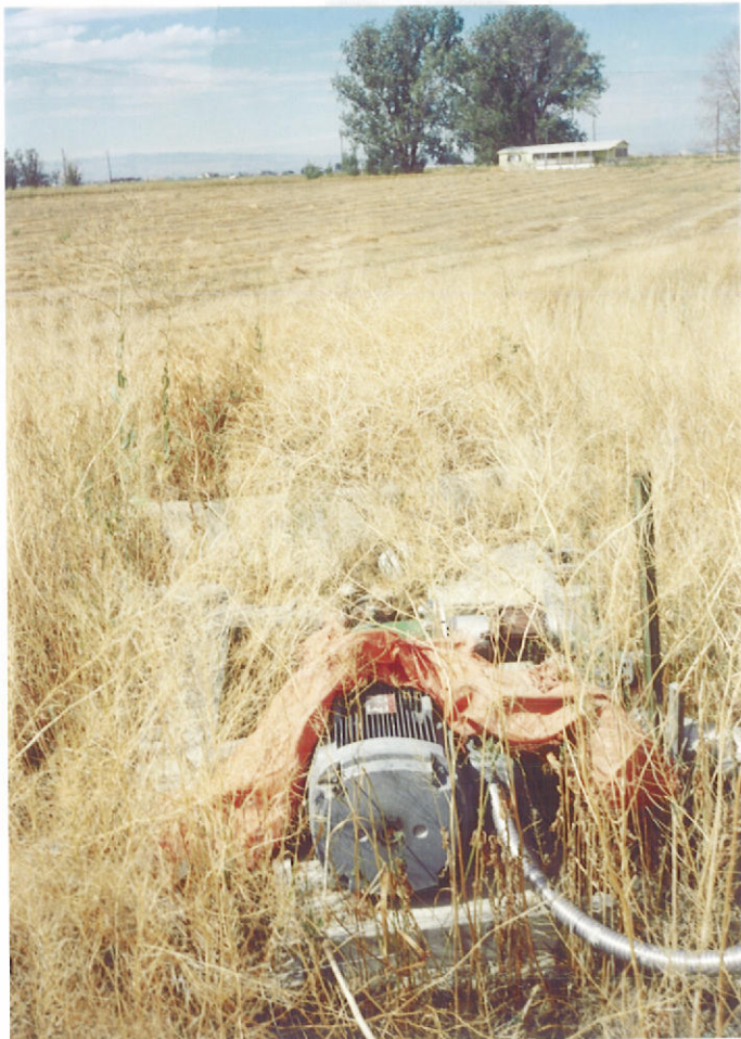
#5 Surface water pump
