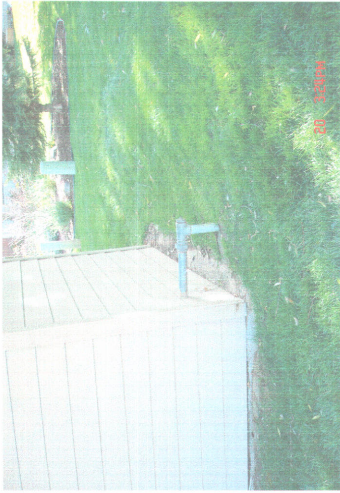
4in Pipe facing Pump House
