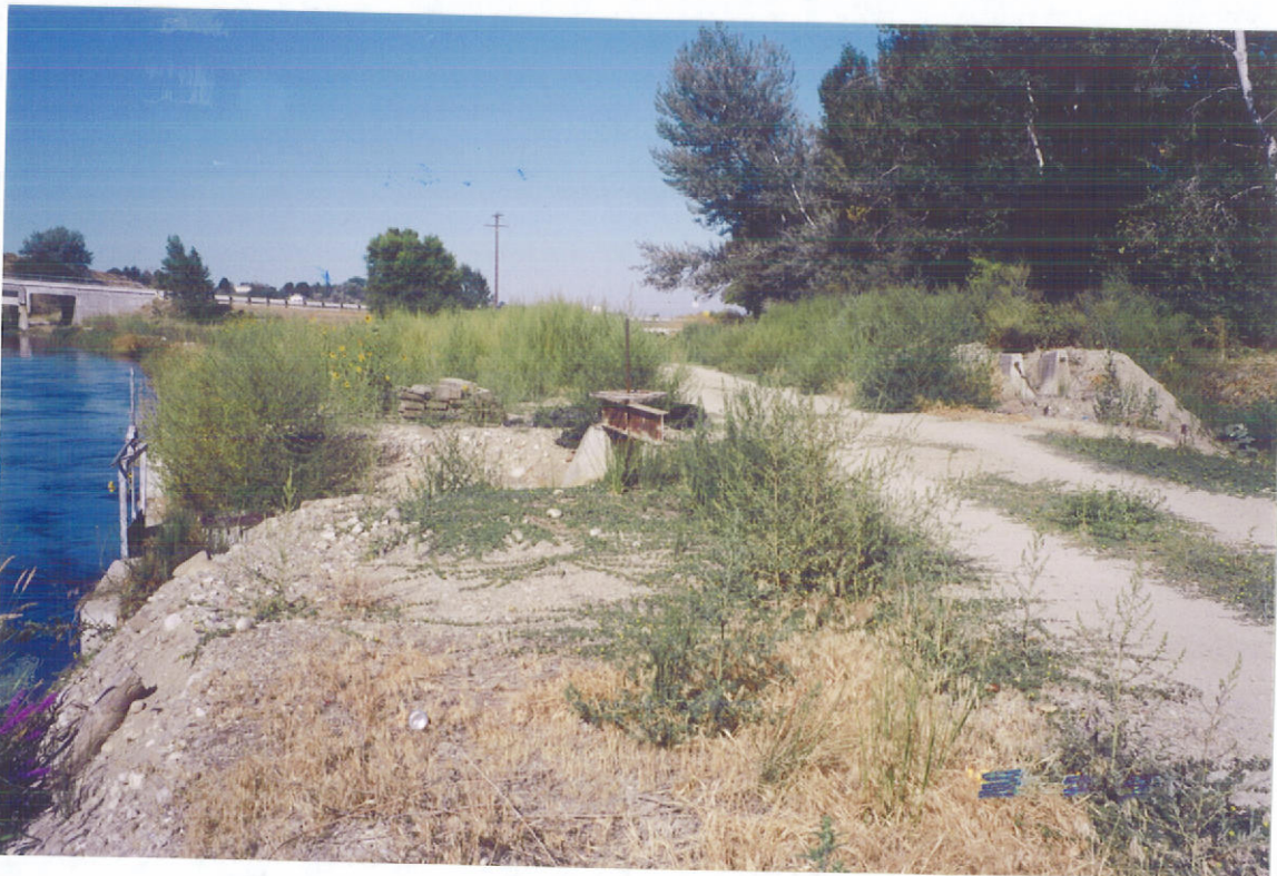
DIVERSION HEADGATE FROM THE PHYLLIS CANAL INTO THE EUREKA CANAL
