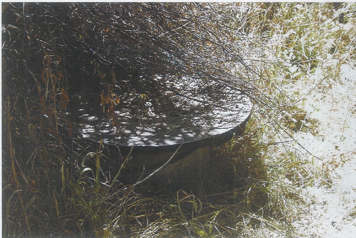
Photo 1. FX Sept 19, 2001. Photos by RDH. Photo of point of diversion, T02N, R07E, S10, NWNE. Cement tile, 3 foot diameter in spring.
