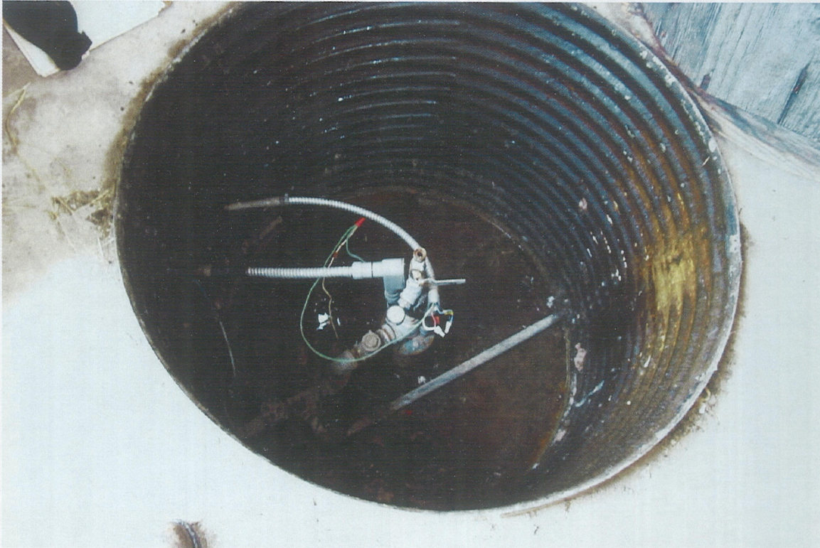
Inside pumphouse. Well used for domestic and commercial purposes (csaxton 2/13/02).
