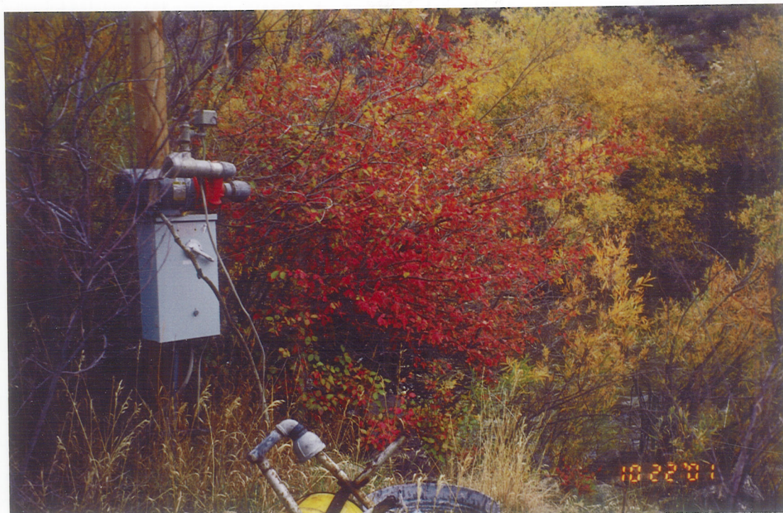
PHOTO # 2 UPPER POINT OF DIVERSION SITE AT THE 5 HP PUMP & MOTOR
