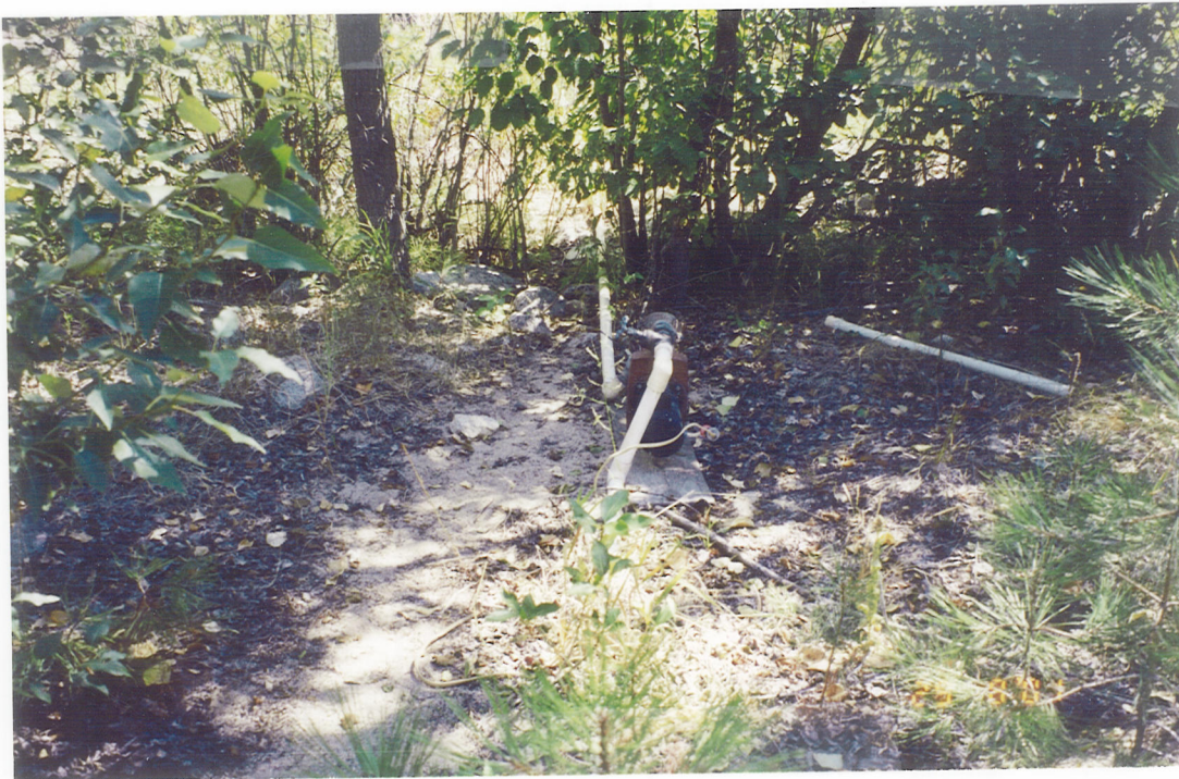
PHOTO #2 PUMP ADJACENT TO THE POD
