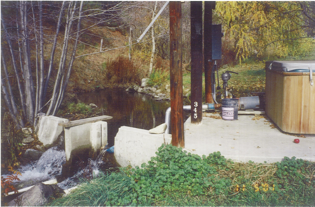
PHOTO # 1 POINT OF DIVERSION— PUMP SITE IN THE SEnw, SECTION 30
