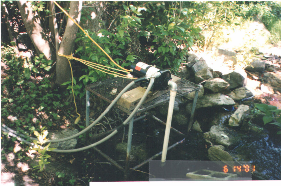
PHOTO #1 POD & PUMP
