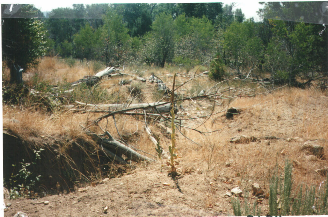
Runoff channel, No diversion, could drain to streamchannel shown above.
