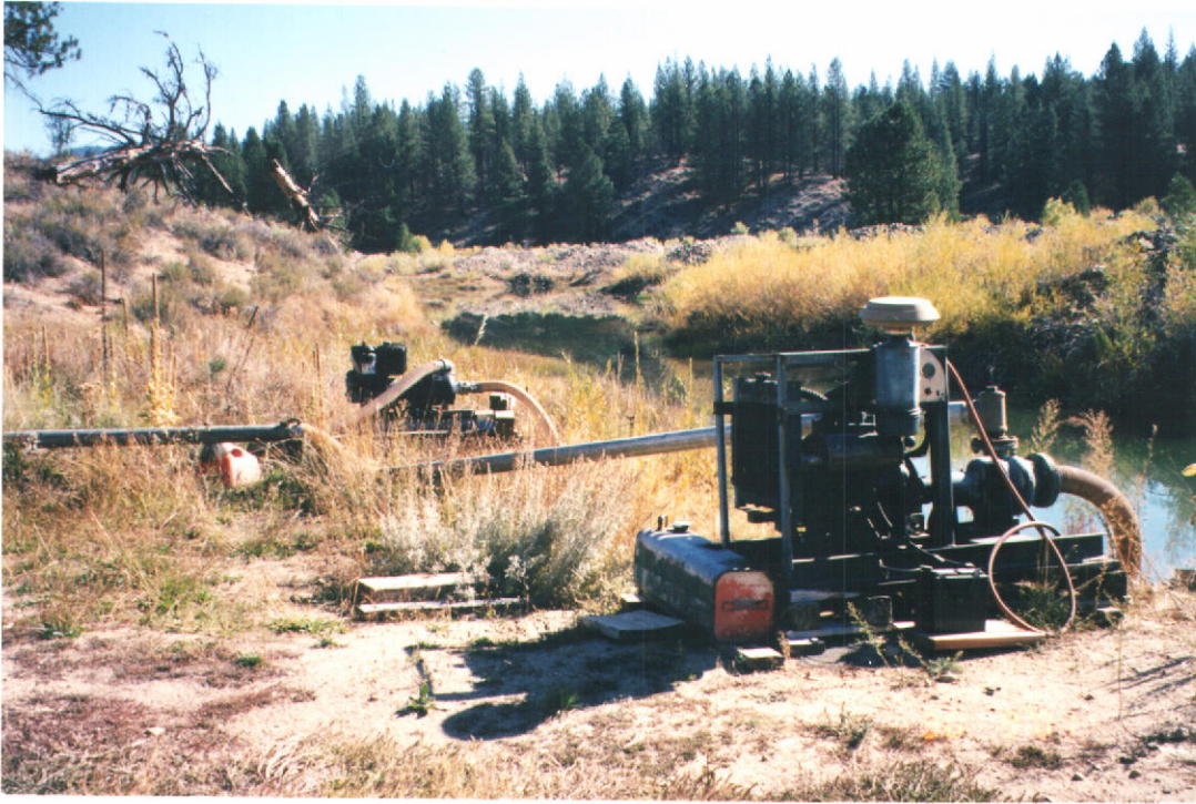
PHOTO #5 PUMPS USED IN THE MINING OPERATION
