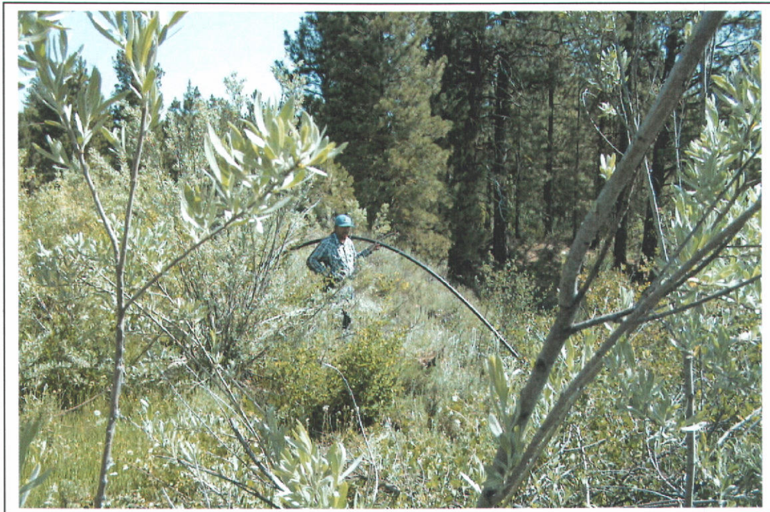
Photo 2. Flexible pipeline 2 inch and 1-1/2 inch. Goes under road culvert and then lays on top of ground and open flow into pond.
