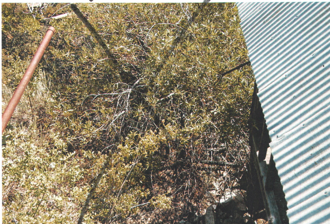
Photo 6: Black pipe on right side of photo from wood tank into Mill. Storage tank has broken into pieces
