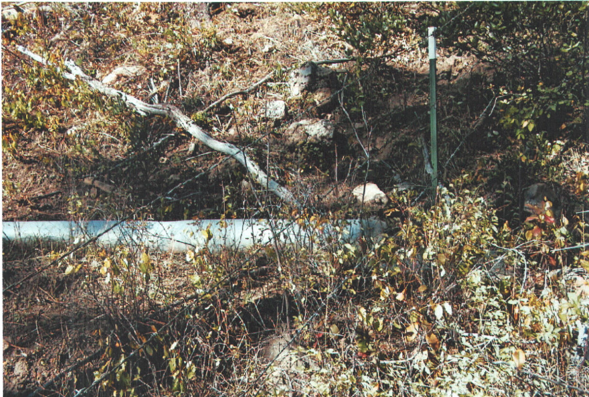
Photo 3. Small culvert used at property line below POD \frac{1}{4} \frac{1}{4} line to prevent washouts.
