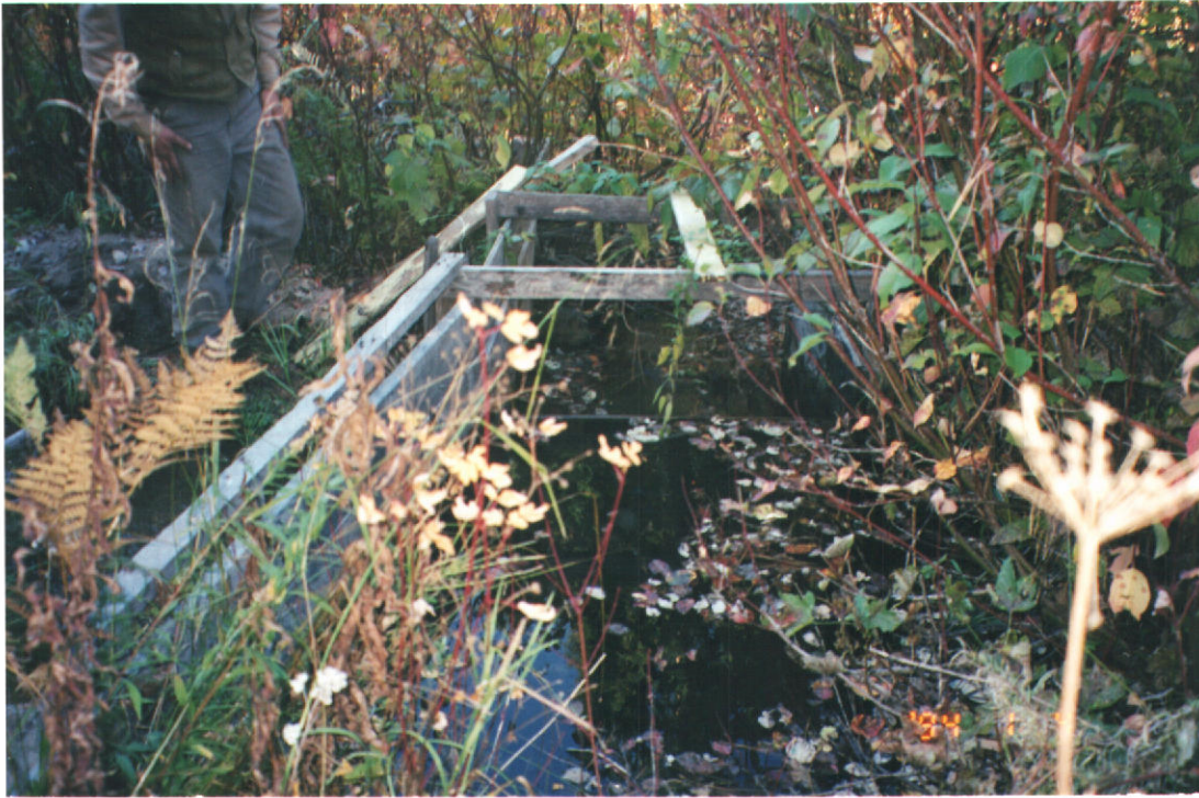
PHOTO #3 DIVERSION STRUCTURE THAT TAKES WATER FROM THE DITCH TO A PIPE TO THE PLACE OF USE
