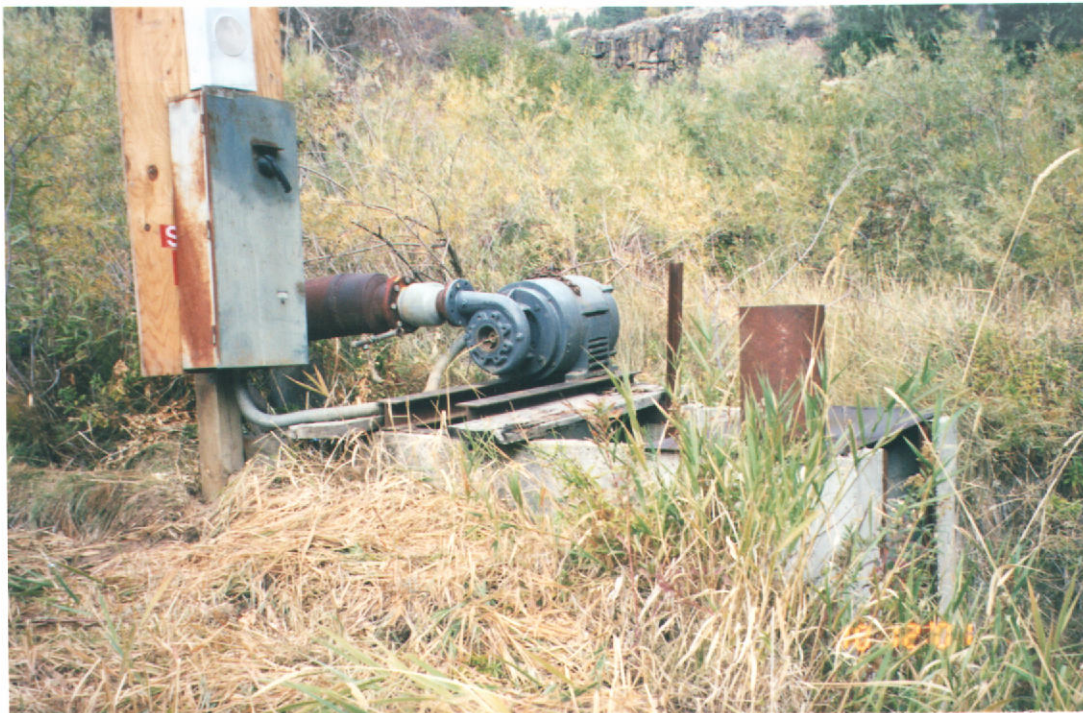
PHOTO #2 PUMP & MOTOR AT THE POD
